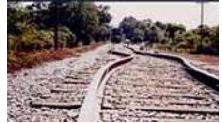
■ Heatwaves can cause railway lines to buckle, causing transport chaos
